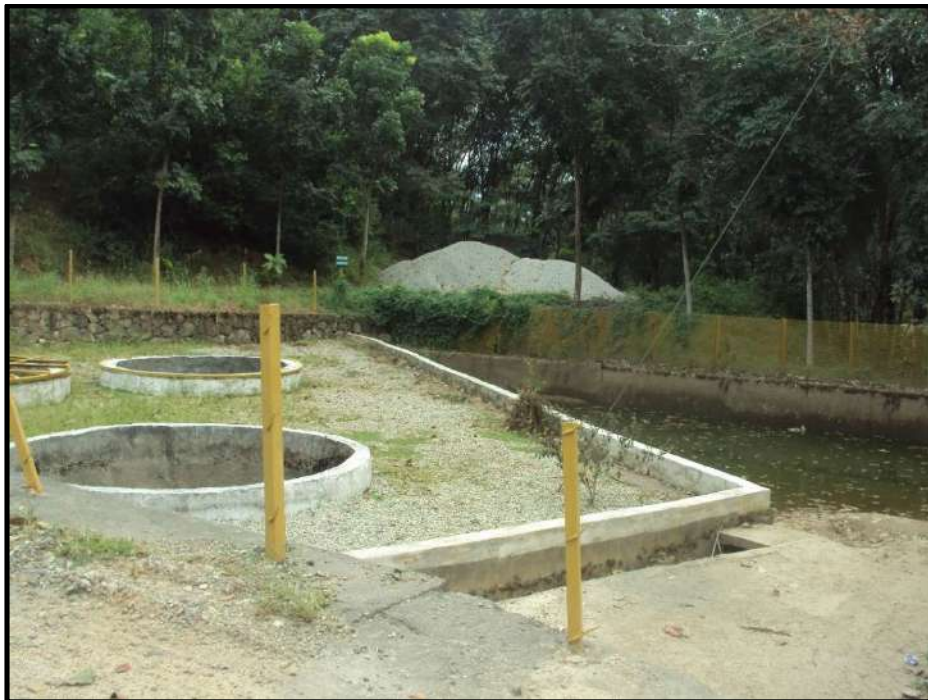
Photographs showing the rainwater harvesting system in the project area
