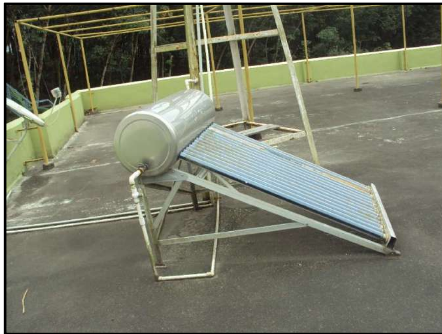
Photograph showing the Solar Energy device installed within the project area
